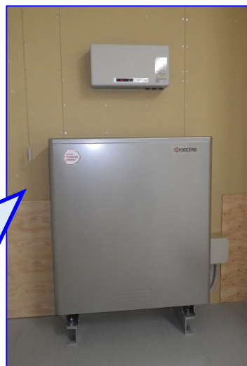
Lithium-ion storage battery connected to solar panels (Rokujizo store)
